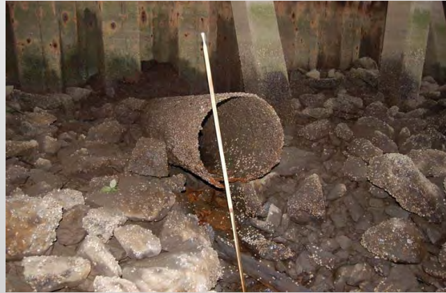
Ponded water in the pipes
