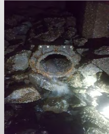
Missing tide gates
